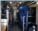
OAO «Deneb» – an ultrafiltration facility with capacity 20 Cbm/ h
