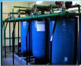
Ion change softening facilities
