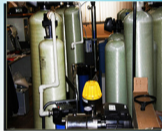
Automatic filling filters section
