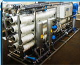
Reverse osmosis facility
